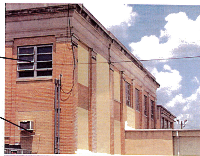
Windows on the south facade are sealed up and stuccoed over where the jail was once attached in the late 1950s
