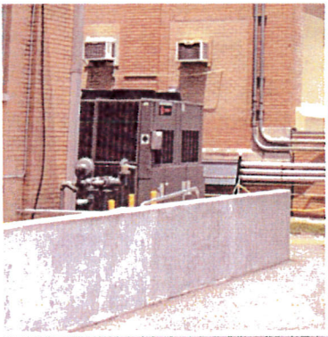
A large air conditioning handler
