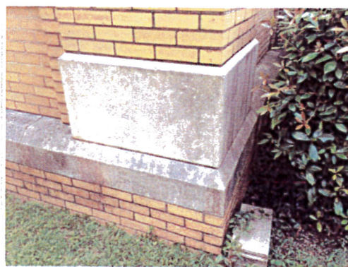
Vegetation growing close to the building
