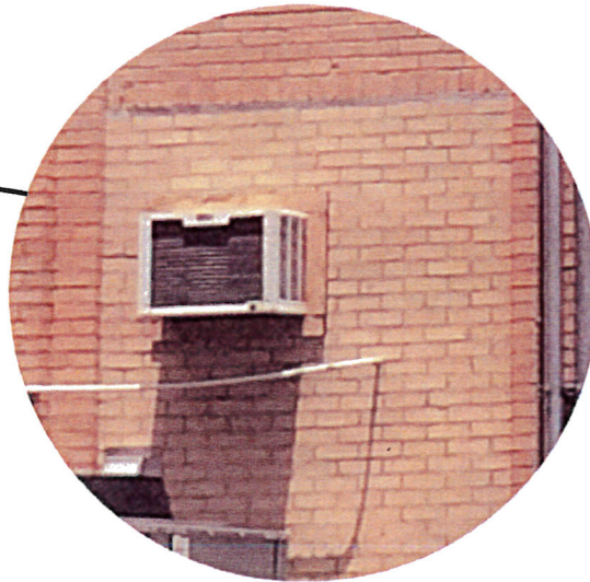
A window unit A/C without a window
