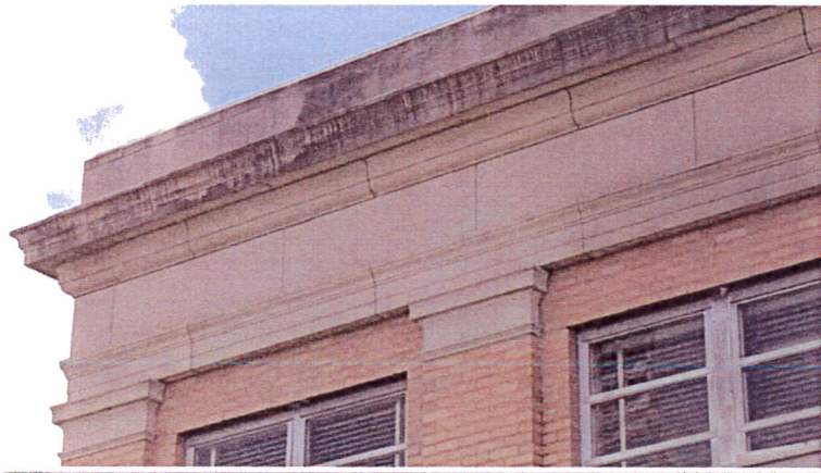
The courthouse's stone parapet is badly stained and in need of cleaning
