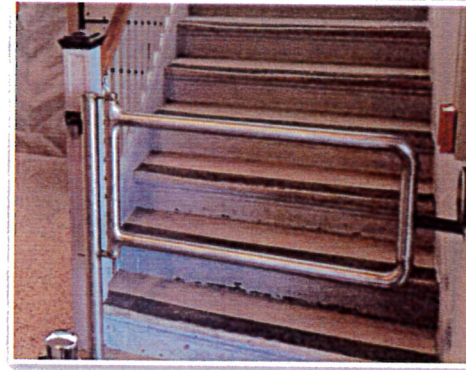
This automated gate was installed recently to prevent access to the second floor without passing security
