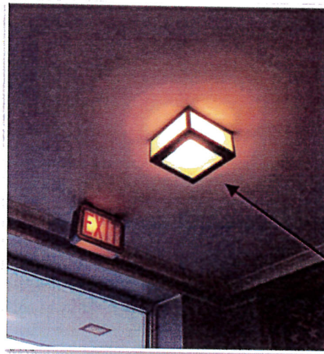
A more distinctive style fixture by the north entrance
