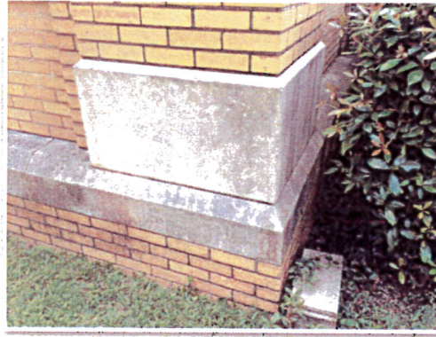
Vegetation growing close to the building
