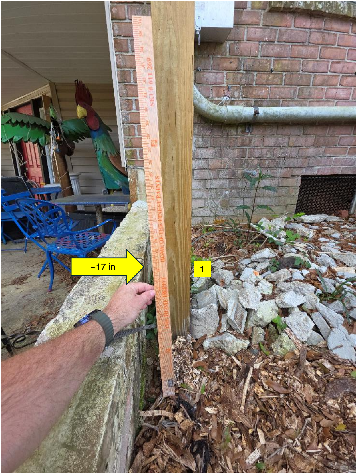
(1) Top wall of patio where fence will be erected. The cement block wall for the basement patio is 17 inches above ground on the outside, along where the fence will be located.
