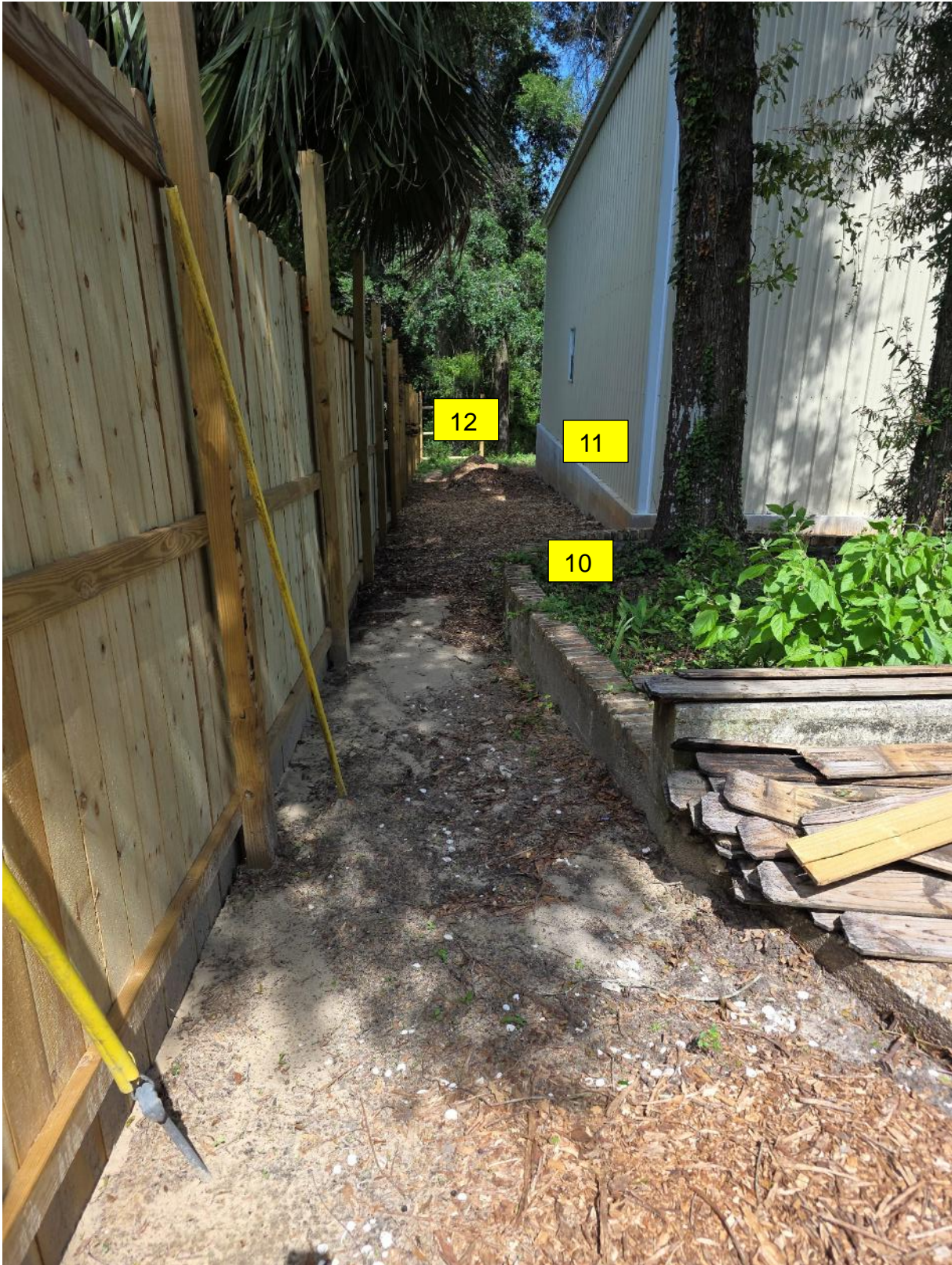
Picture shows front upper(10) and rear lower(11) corners of garage slab height.
