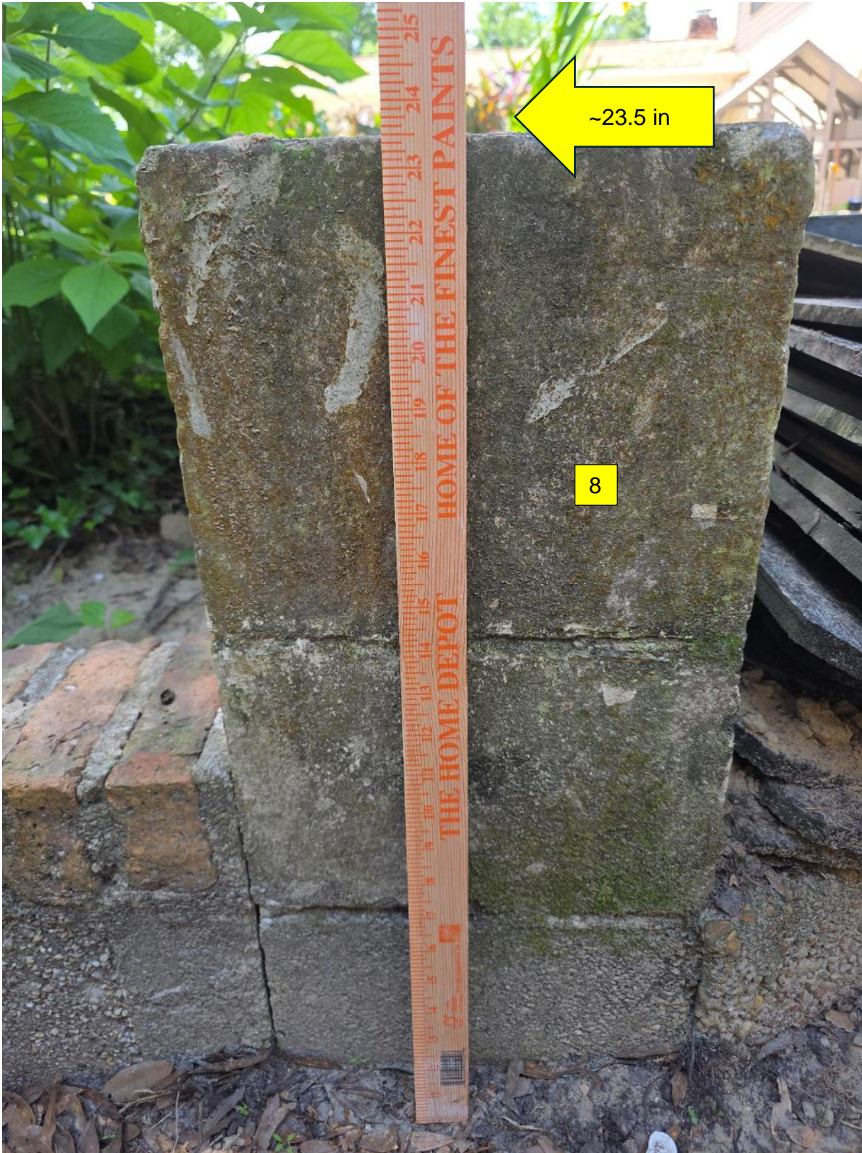
(8) view at end of block wall, near the edge of the patio near the fence location.
